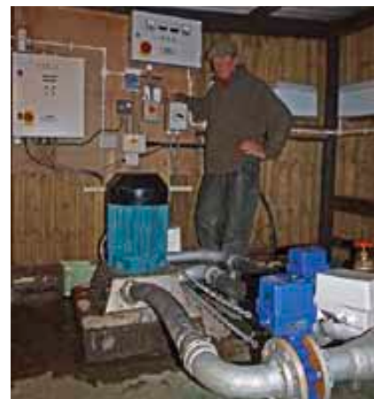
Neil Gourley with the 12 kW hydro generator - one of two systems installed at Auchencheyne with the help of farm labour.
